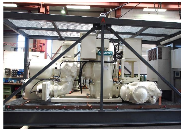
Fig. 6. Gas-insulated power switch located in the outdoor part of the measurement container
